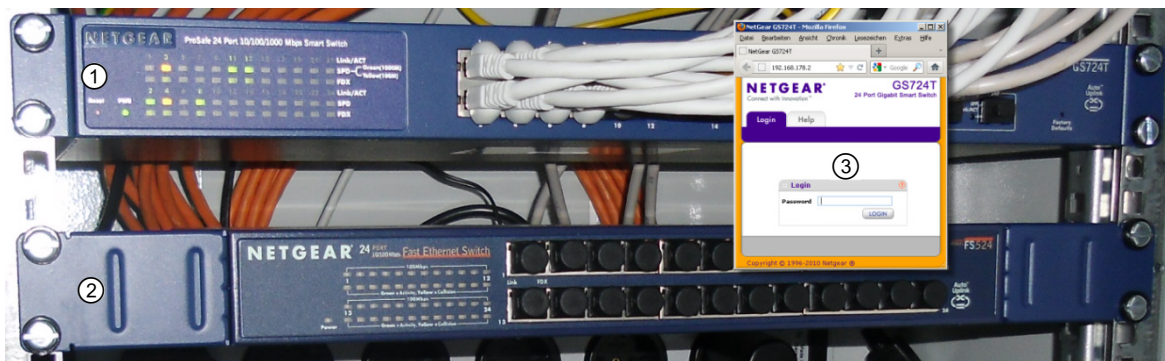
19"-Switches: Managed ①, Unmanaged ② und Webinterface des Managed Switches ③
